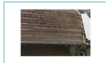
Dirty Air Conditioner Indoor Unit
